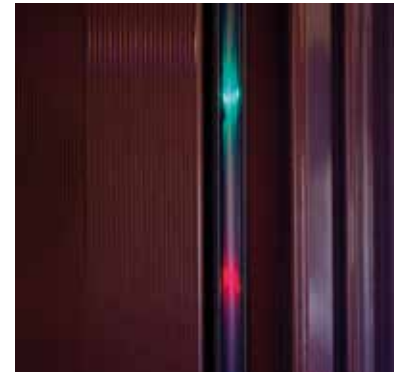
Infrared sensors all around the perimeter for entry/exit from the cabin, to guarantee full safety.
